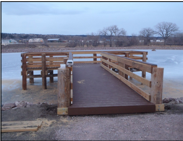
A little work on the approach to the deck and this wheelchair accessible fishing pier at Black Elk Pond in Newcastle will be ready for anglers.
