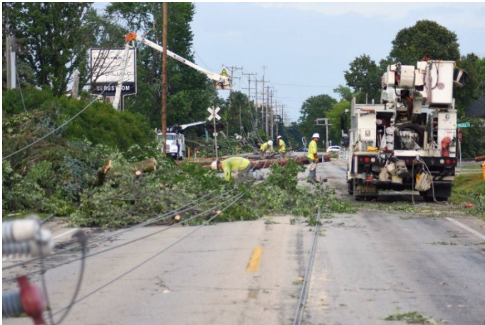
WE Energies crews are working to restore power in Outagamie County. Courtesy: WE Energies.
