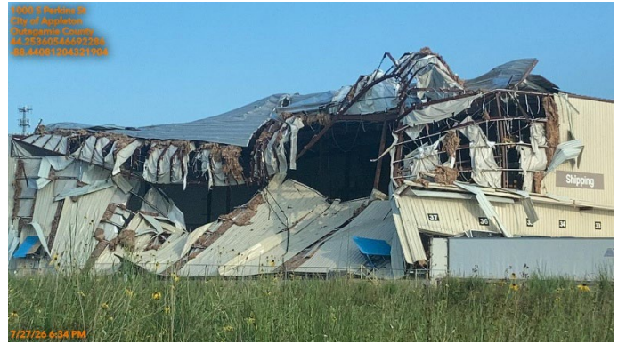
Damage at Miller Electric in Appleton.
