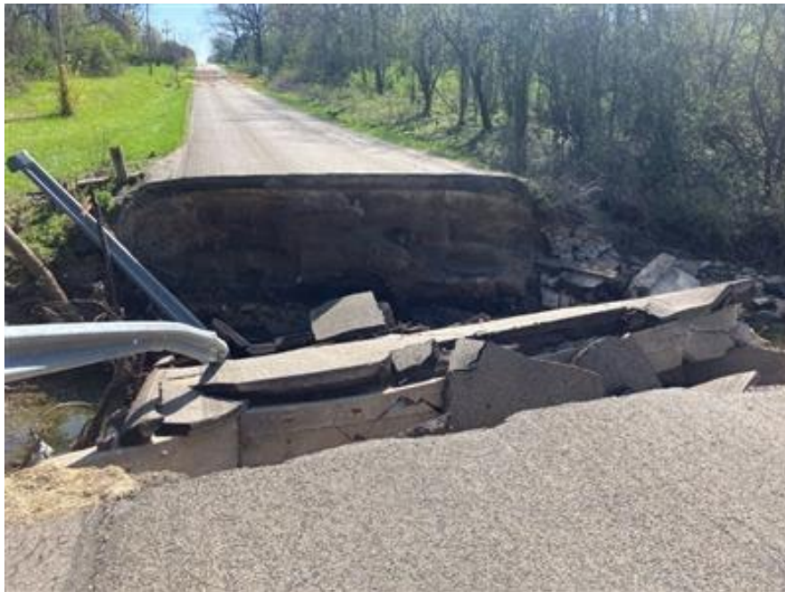
Photo: Bridge damaged by flooding in Rock County, WI.
