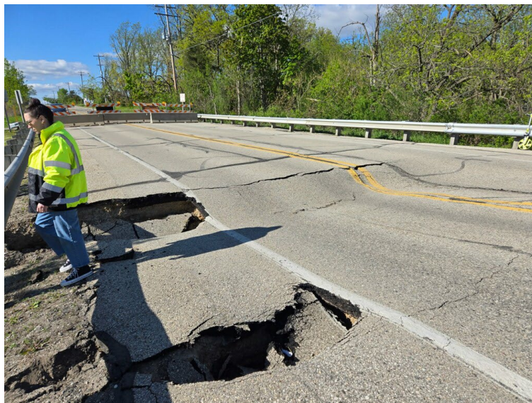
Photo: Road damaged by flooding in Racine County, WI.
