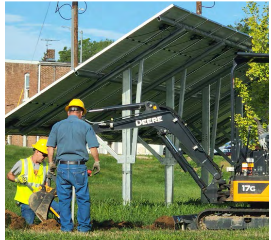
Installation of Electric Vehicle Charging on Western Technical College's Campus. Photo Credit: Xcel Energy
