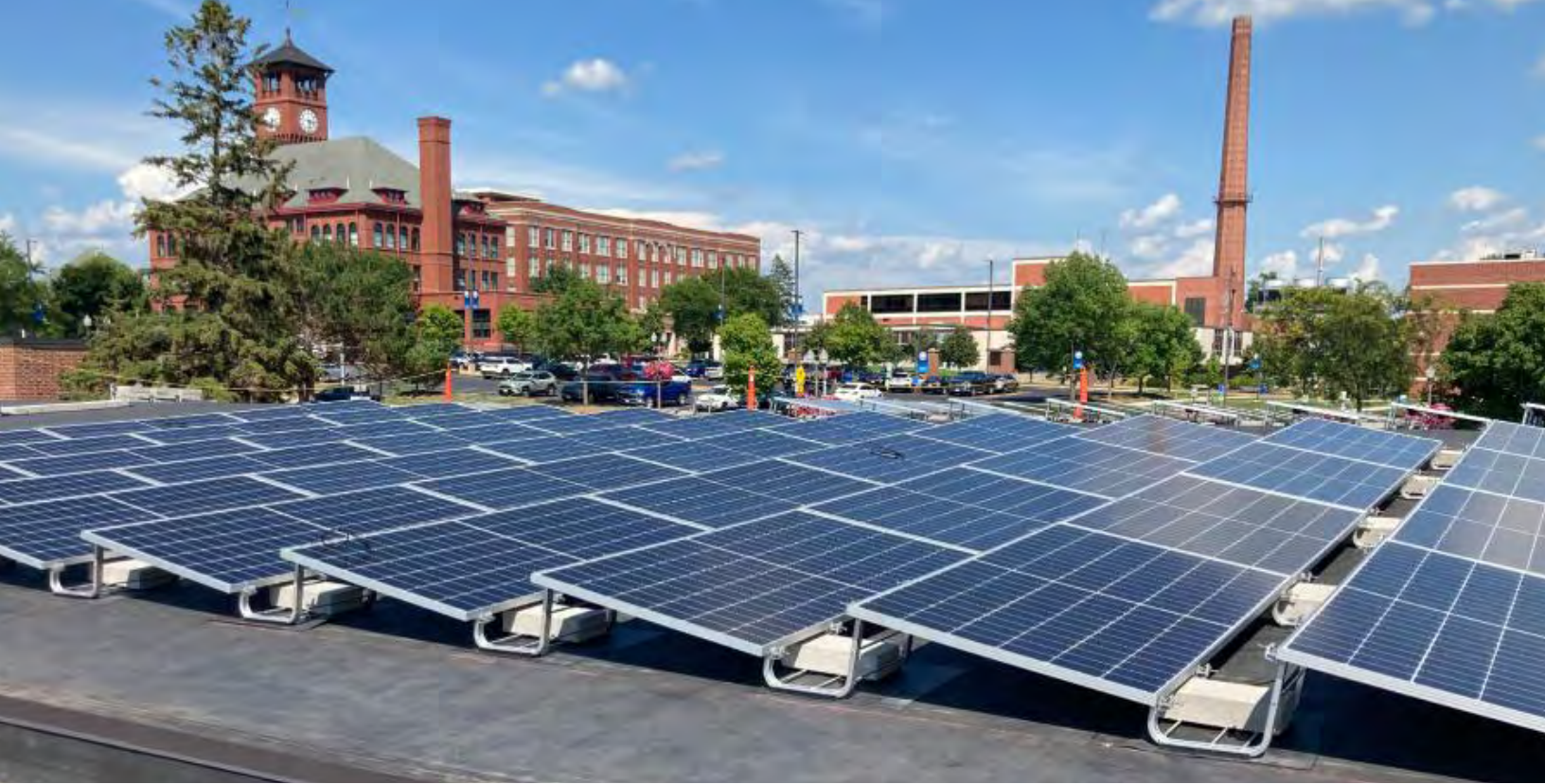
UW-Stout General Services Building solar panel array
