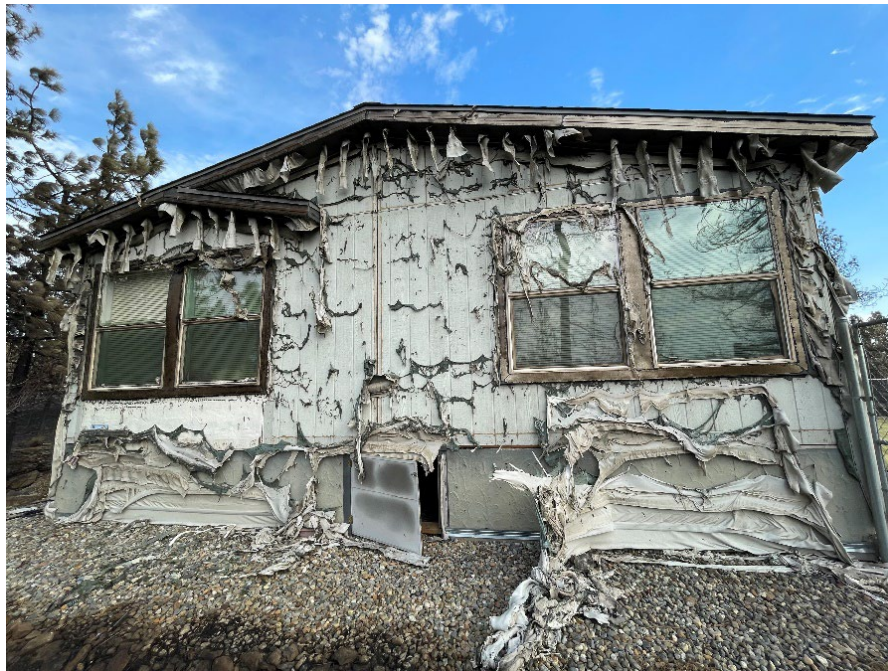
Figure 7. Melted siding on a home in the city of Medical Lake following the Gray Fire. Photo taken during the state Preliminary Damage Assessment August 2023.
