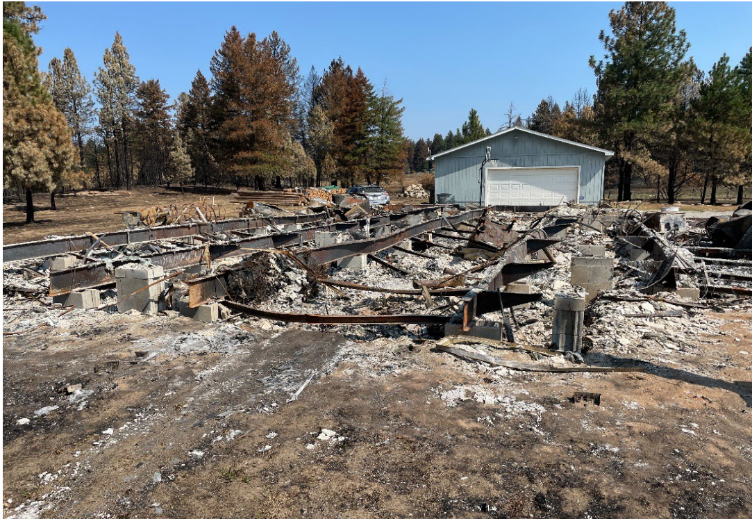
Figure 3. The foundation and a garage are all that remains of a home destroyed by the Oregon Road Fire in the rural community of Elk. Photo taken during the state Preliminary Damage Assessment August 2023.
