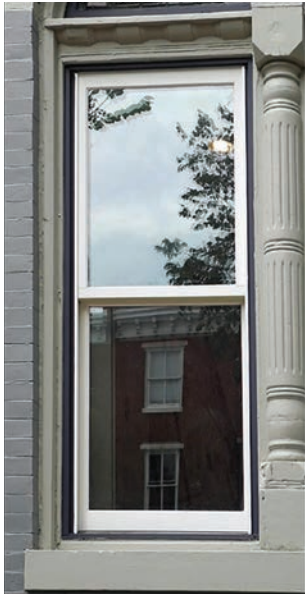
Aluminum clad wood window replacement intended for rough opening installation but here inserted within an existing jamb.
