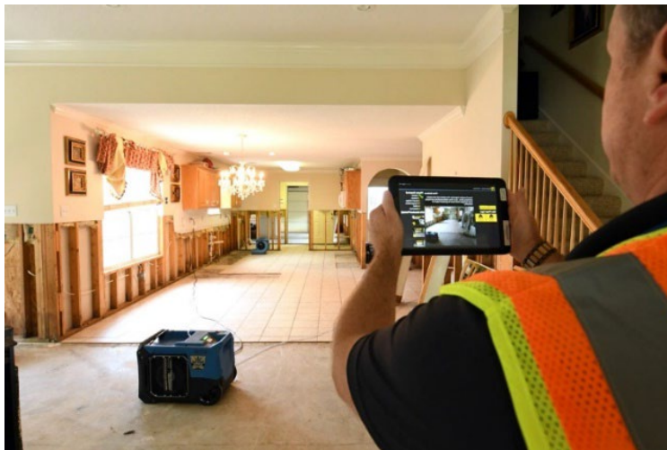
Figure 1. An inspector documents damage to a home after a significant flood event
