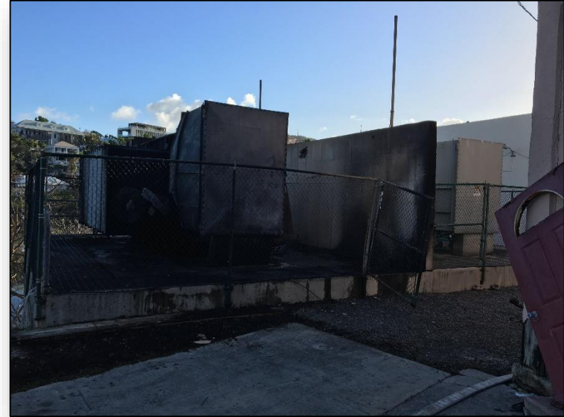
Burned sub-station on St. John Photo Courtesy of FEMA Region II
