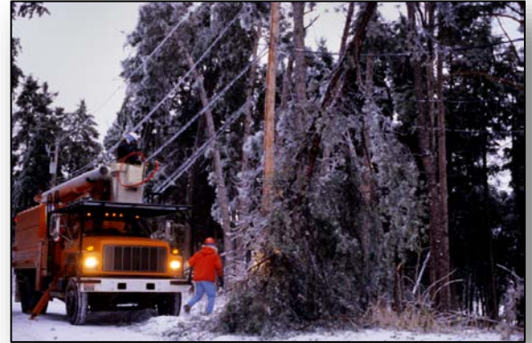
Photo Courtesy of Oklahoma City Public Power
