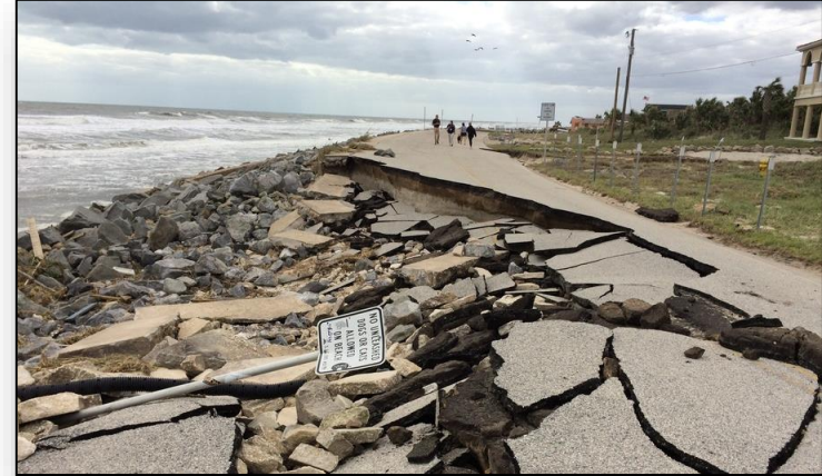
FEMA Officials Survey Damage on Highway A1A near St Johns county Photo Credit: Eileen Lainez
