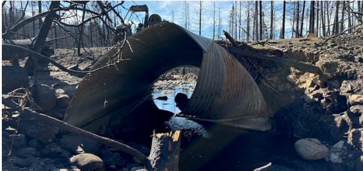
Figure 5. Damaged aquatic organism passage (AOP) culvert near milepost 11.8 on NFS Road 625.
