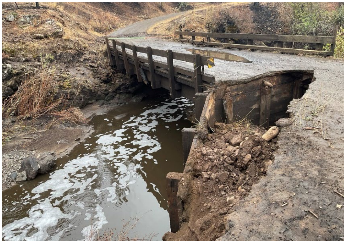
Figure 4. Photo of the Chief Eagle Eye Creek Bridge taken after the post-fire flooding
