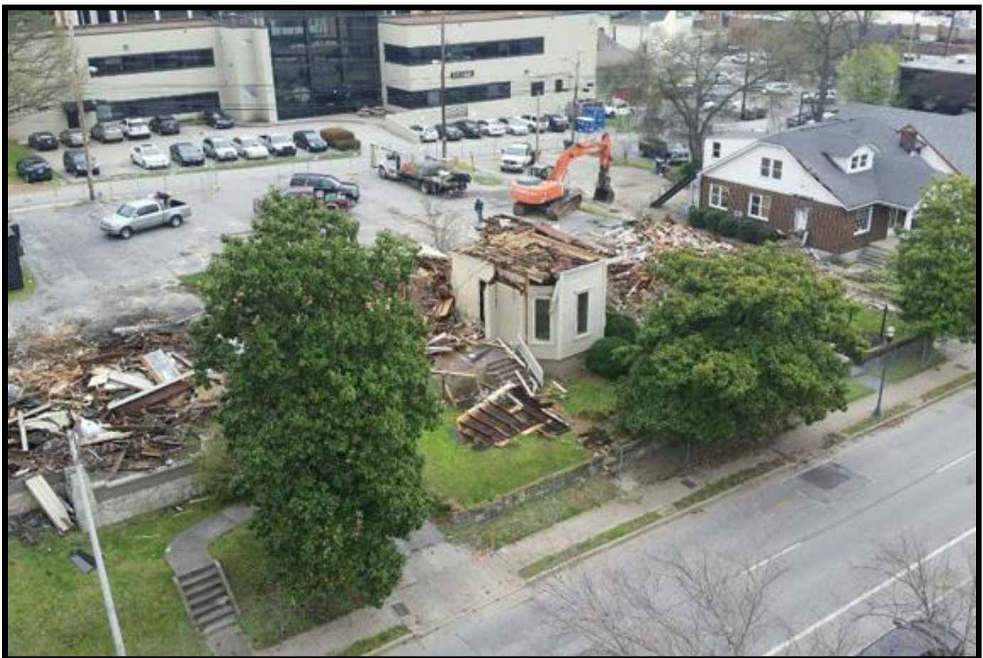
Figure 25. Demolition of five historic houses adjacent to SESAC on Music Row in March 2015 for redevelopment into a luxury apartment building. Photo by Victoria Lazarus.
