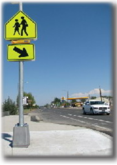
U.S 730 / 1 st St. flashing beacon
