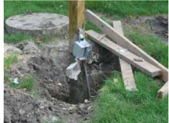
Flood damaged SSTS electrical box
