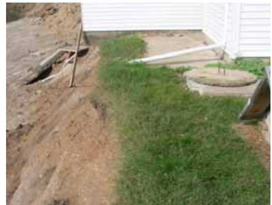
Washed away SSTS in eroded stream bank
