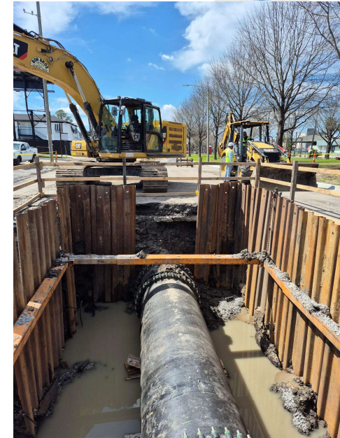
Saturday February 28 Water main returned to service Roadway full returned to service on Sunday morning (March 1)
