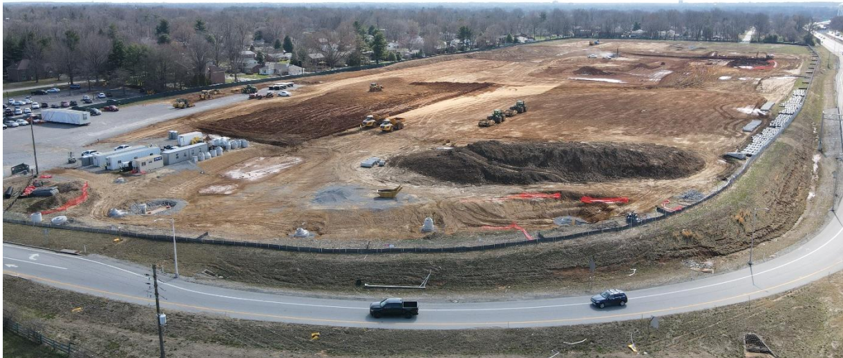
Drone view of the construction site of the new Louisville VA Medical Center in Louisville, Kentucky, on March 15, 2022.
