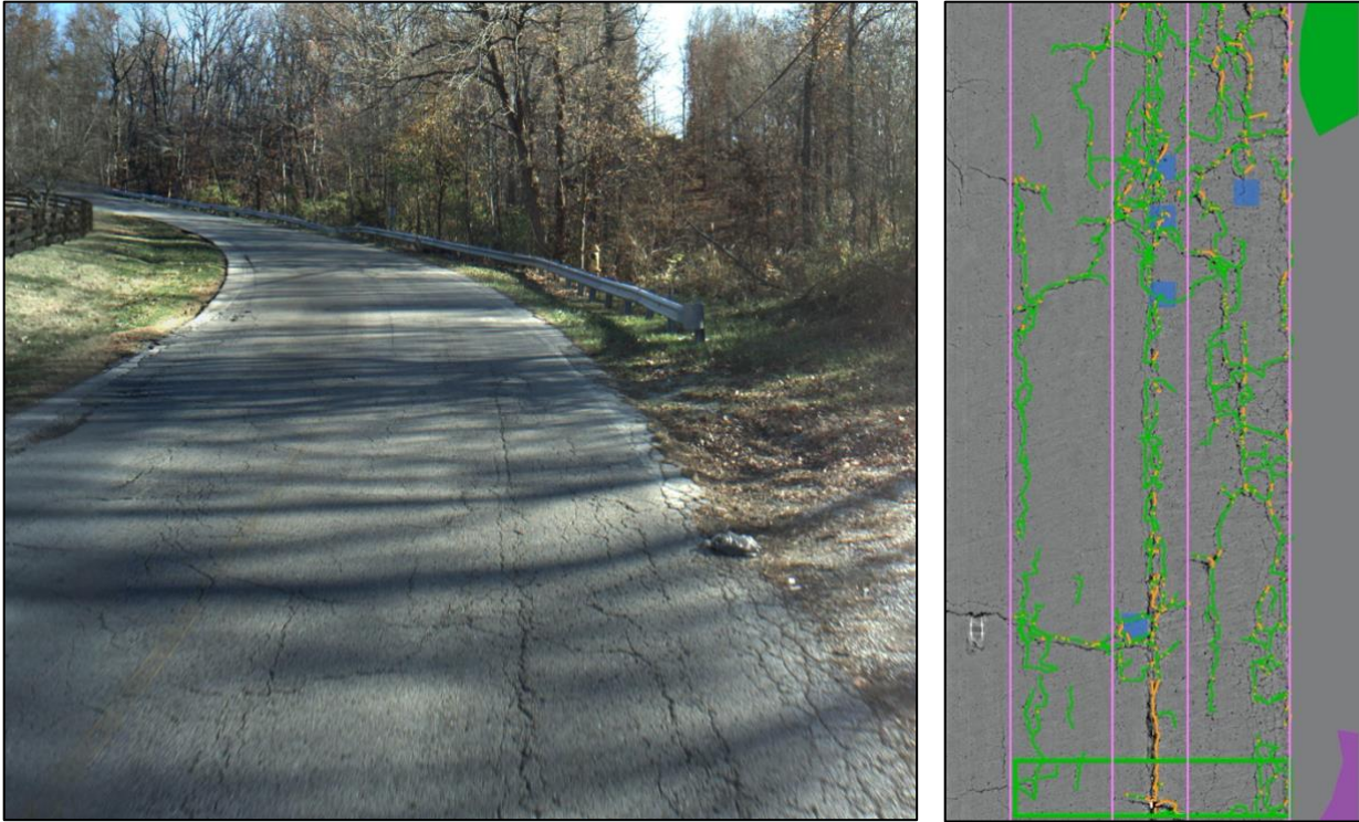
Figure 5.2.3.a : Mandli Right of way (ROW) imagery of a road with a PCI score of 28 , which is classified as Very Poor (Left). Figure 5.2.3.b : Image of the LCMS Rage Downward Image with Overlay of the road depicted in Figure 5.2.3.a.
