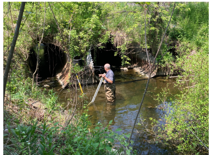
Drain Commissioner, Ken Yonker, inspecting a drain. Photo taken by Joel Morgan.
