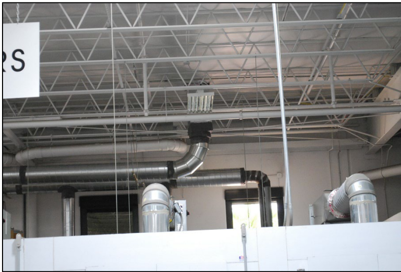
Stack from Scrubber 1
