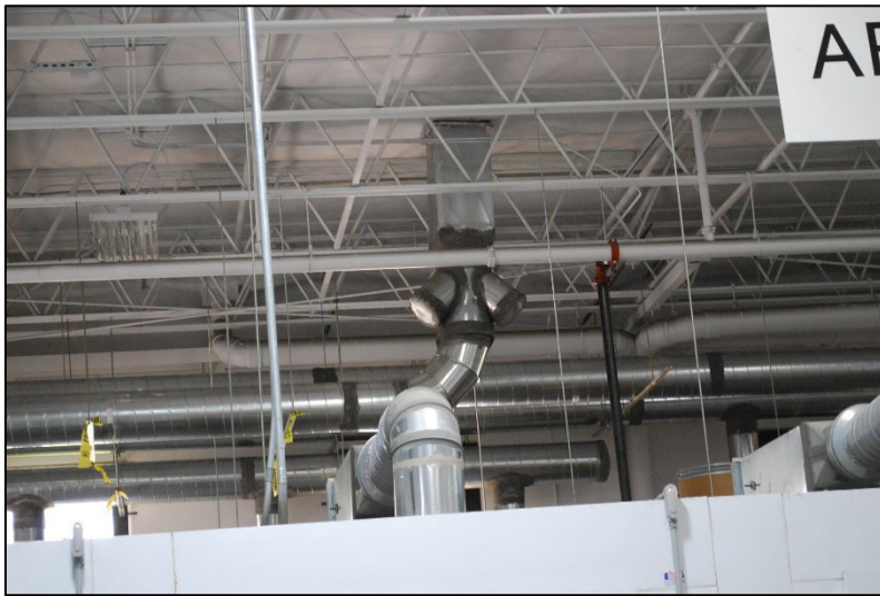
Stack from Scrubber 2
