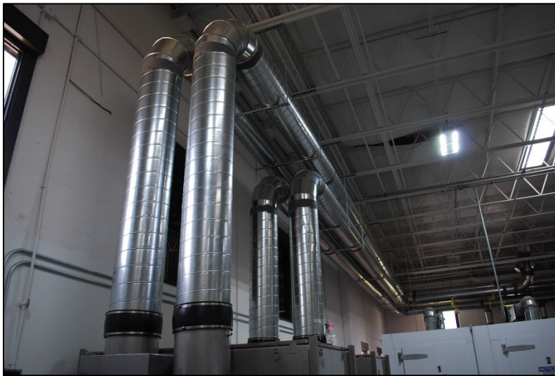
Scrubber Intake and Exhaust Pipes
