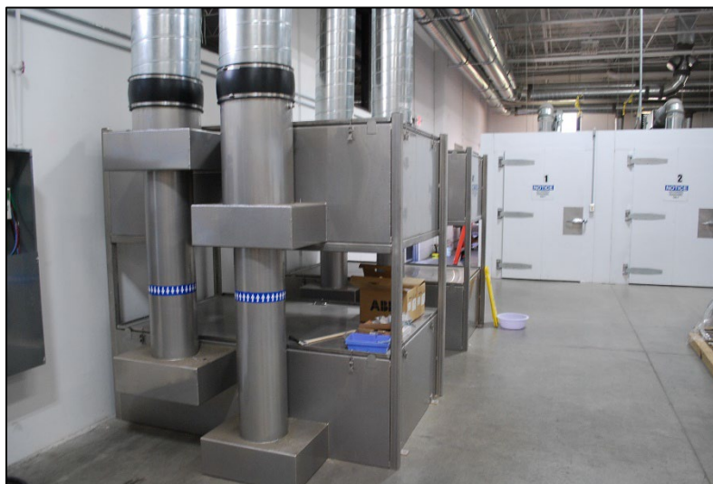
Dry Bed Scrubbers
