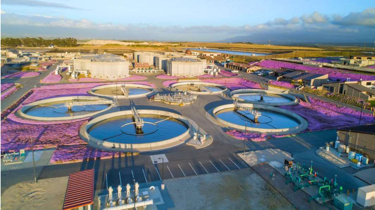
The Monterey One Water (M1W) Regional Treatment Plant is installing codigestion capacity. Photo courtesy Anaergia
