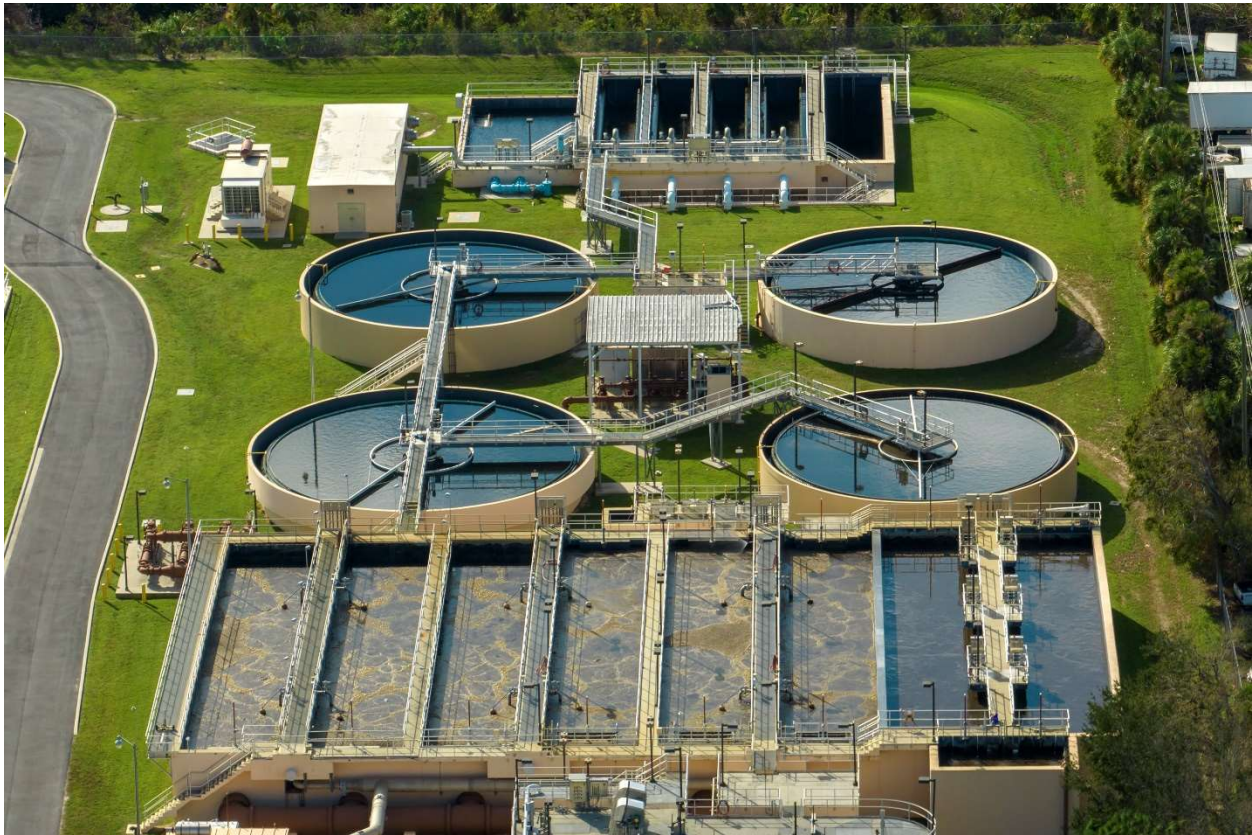
Wastewater Treatment Plant. Image from Istock.com
