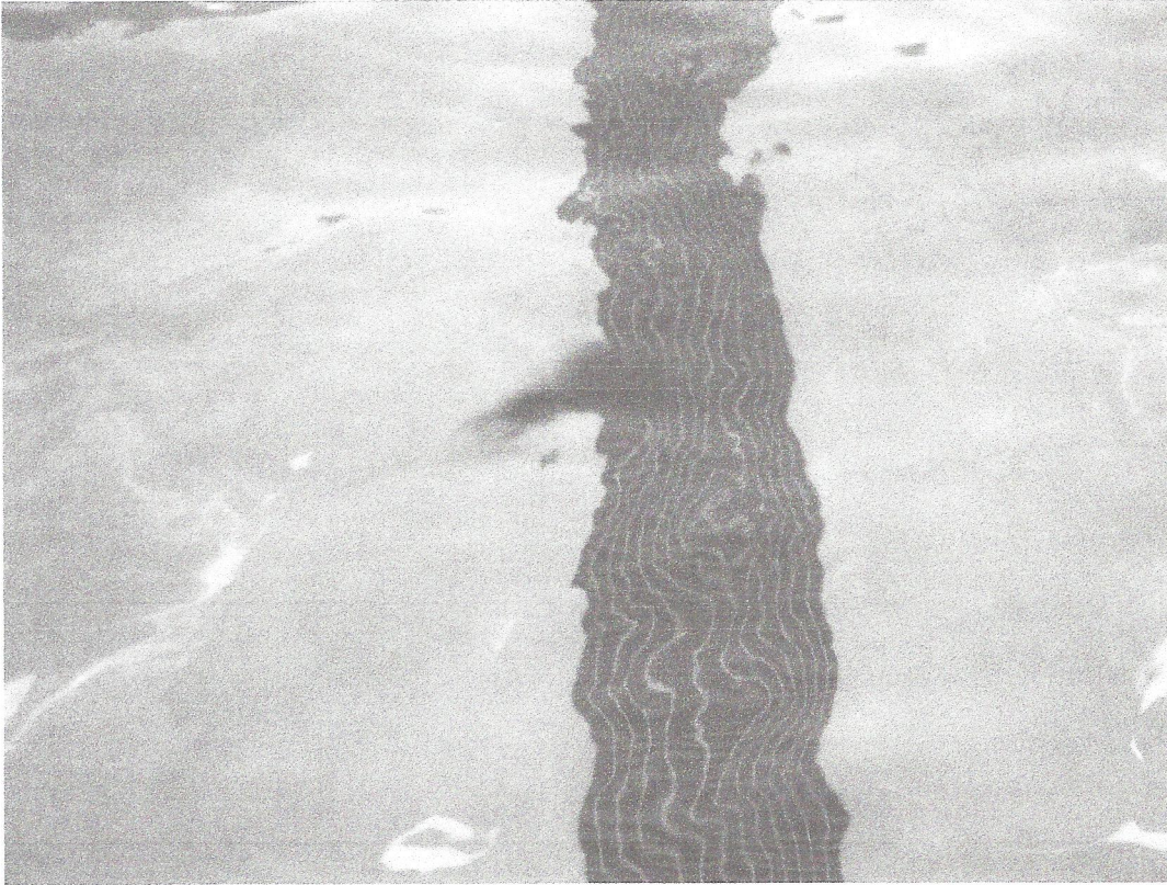
P1: Rust stain on the bottom of the instructional pool.
