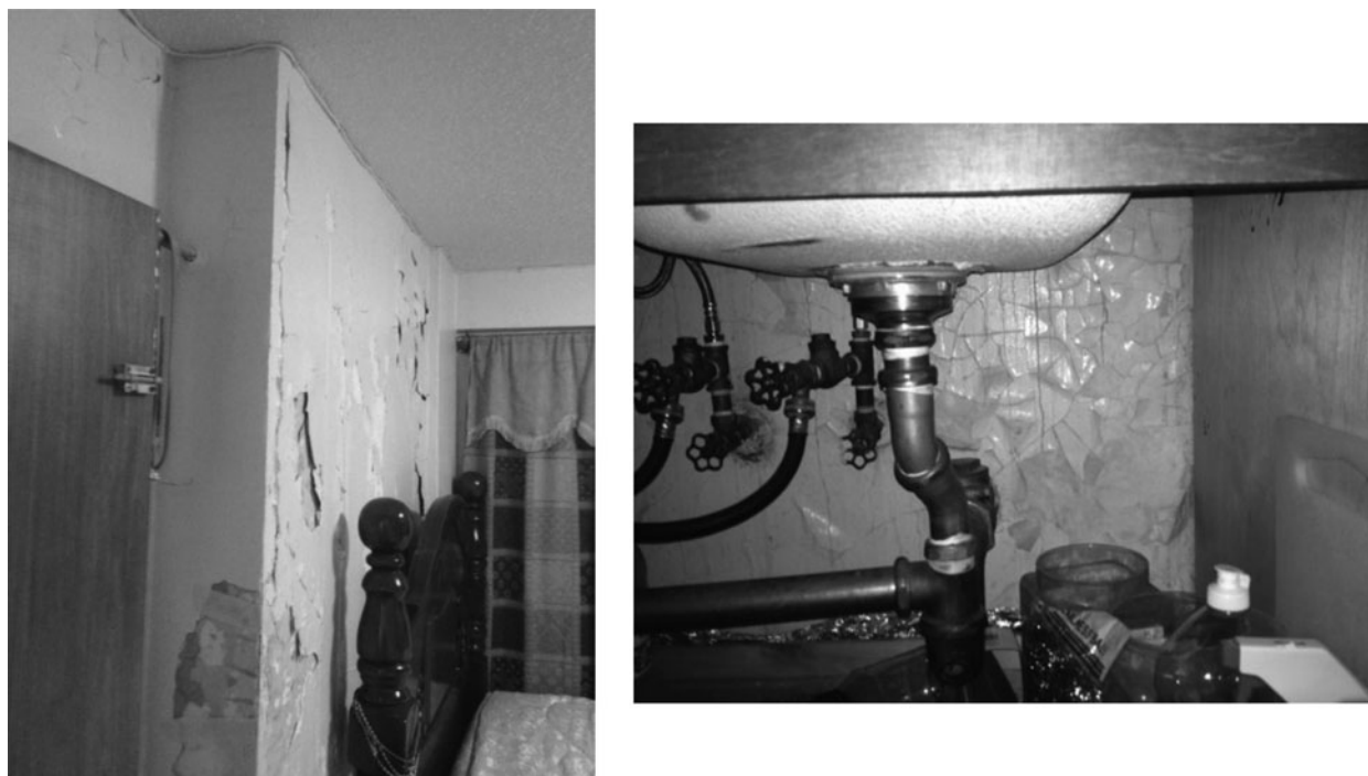
FIG. 2. Housing conditions prior to intervention.
