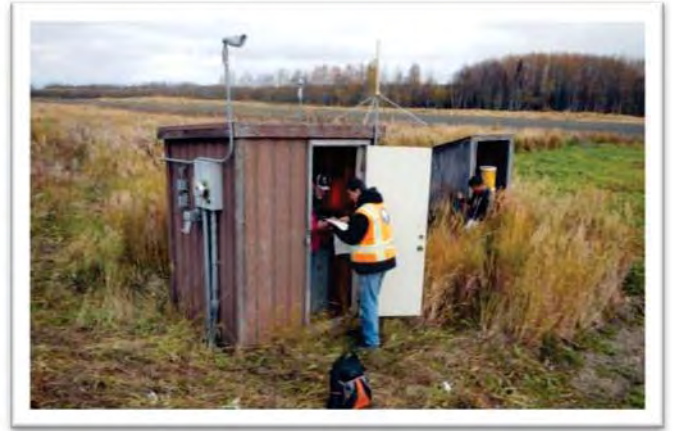
Airport inspection in Holy Cross this past summer. Photo credit - Jason Sakalaskas, DOT&PF
